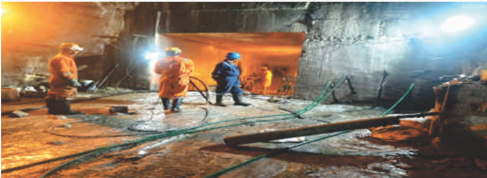
Arresting Leakage of 6500Lit/Min
